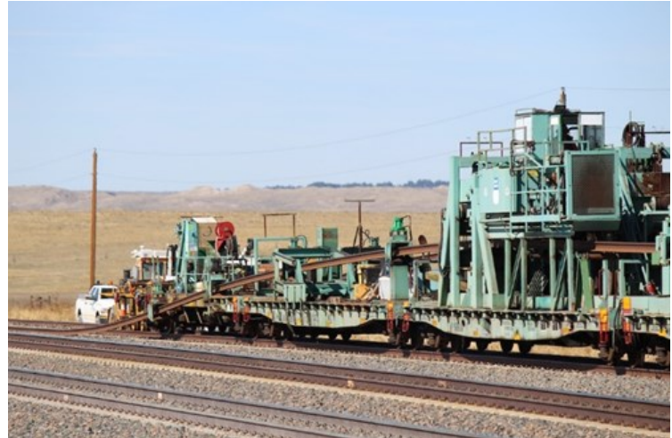
Union Pacific track crews lift one of the rails on the third main track on Myles Hill on the Powder River Subdivision west of Lusk, Wyo., in October 2020. Bill Stephens
