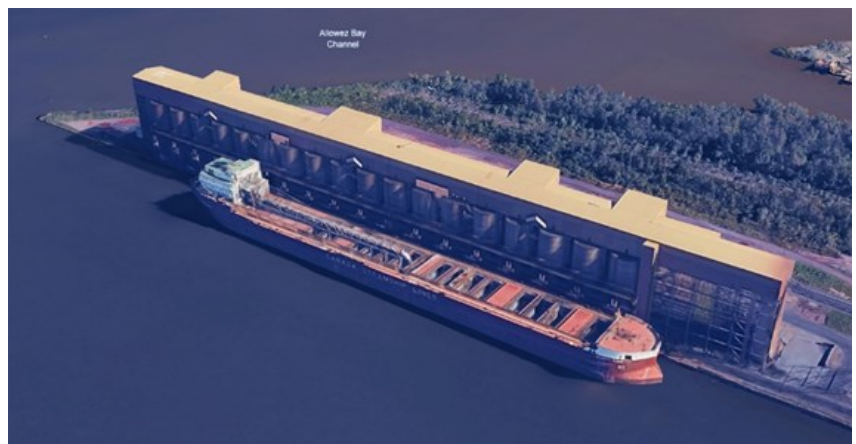
The BNSF Allouez Taconite Loading Facility in September 2024, about two months after it was damaged when hit by a ship. Google Earth
