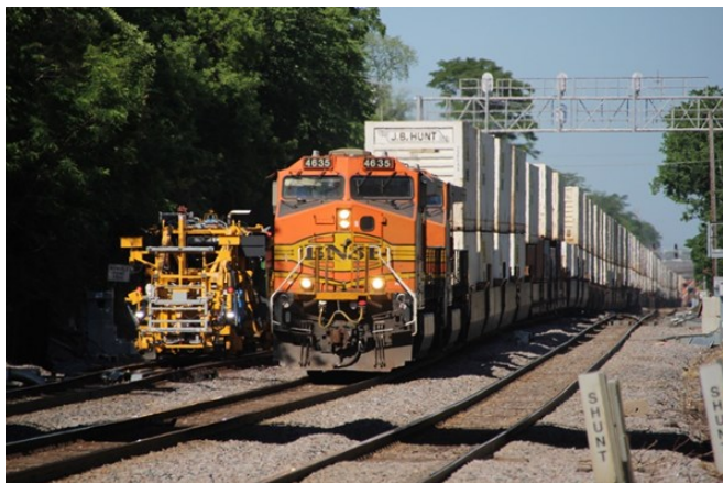
A BNSF intermodal train slows for maintenance work in Hinsdale, Ill., on June 13, 2021. BNSF will spend $2.8 billion on system maintenance as part of its 2026 capital plan. David Lassen
