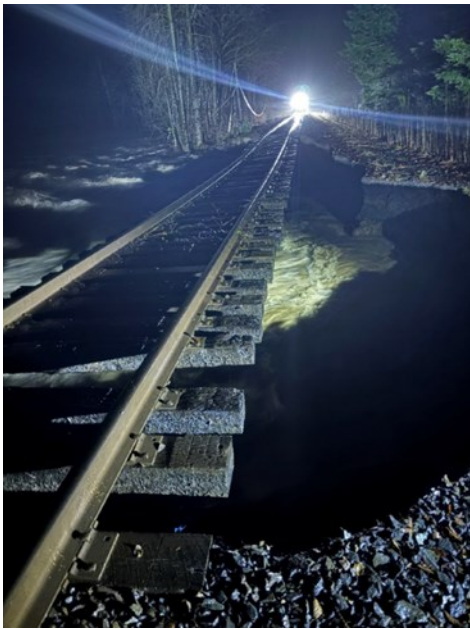
L: BNSF Railway's Stampede Subdivision had a washout at milepost 66 during last week's flooding. BNSF Railway
