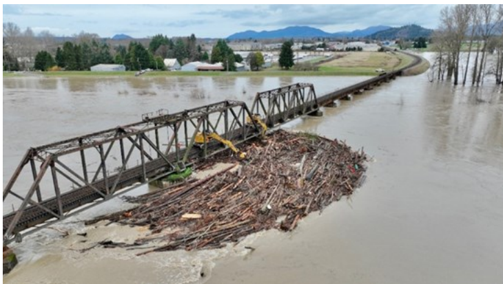
BNSF crews work to keep flooding debris clear around the Mt. Vernon Bridge over the Skagit River in Washington. BNSF
