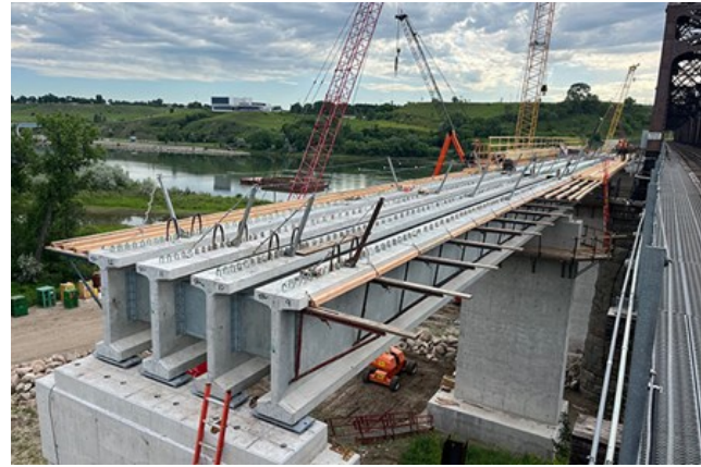
R: Work is progressing to form the deck for three of the BNSF bridge's 12 spans over the Missouri River in North Dakota. BNSF
