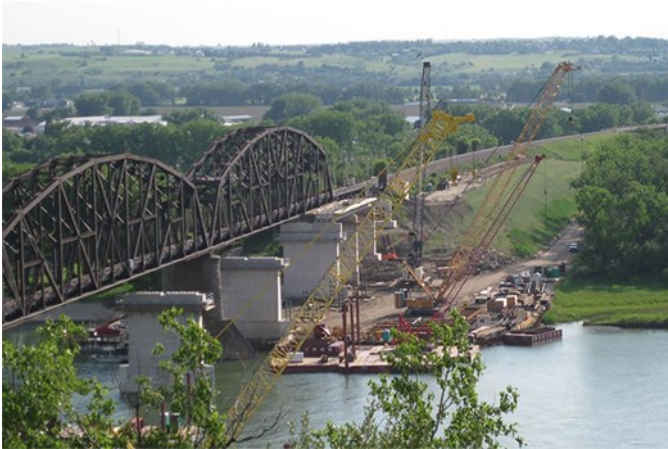
L: BNSF is building a new bridge across the Missouri River in Bismarck, N.D. BNSF
